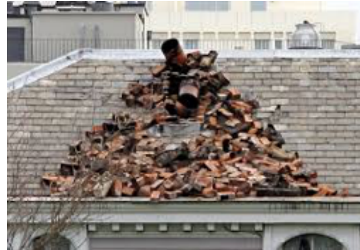
Chimney failure, Christchurch New Zealand 2010 Source: BeckerFraserPhotos, CEISMIC, Canterbury Earthquake Digital Archive
