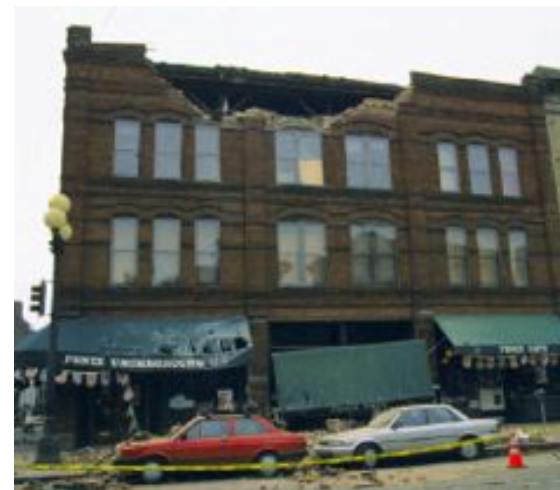
Parapet and wall failure, Source: Earthquake Engineering Research Centre, 2016
